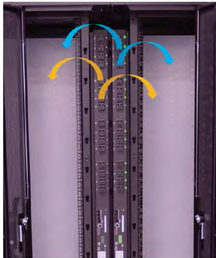
Figure 3: VersaPOD Zero-U space with primary and secondary PDUs shared between two cabinets
